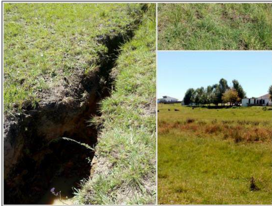
Figure 19 Existing erosion concerns on the mid-slope areas of Mooi River
