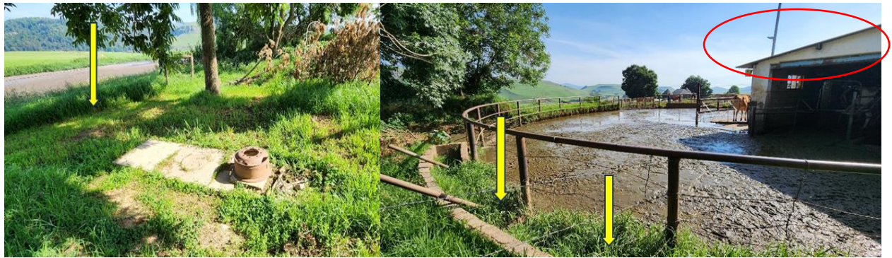
Figure 8-1: Trenches Conveying Sludge from Dairy Area to the Slurry Dams
